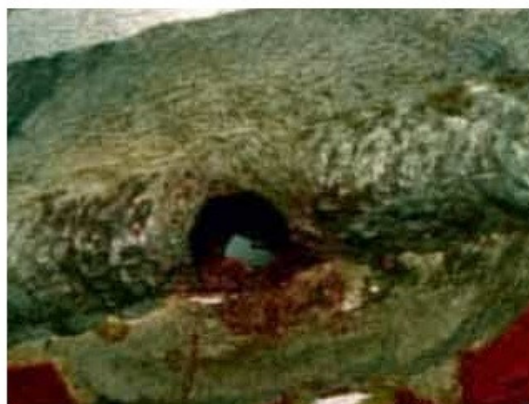
Fig. 3.8: Microbiologically influenced corrosion (MIC) or bio-corrosion
