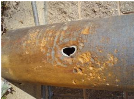
Fig. 1.4: Pitting corrosion of mild steel
