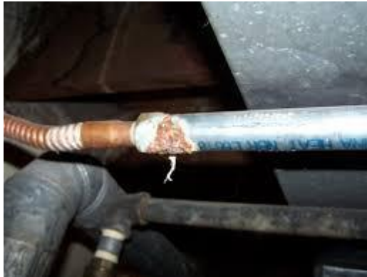
Fig. 1.3: Mild steel coupled with copper showing galvanic corrosion
